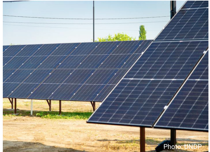
A photovoltaic system installed in Molovata, Dubasari district, with a capacity of 24 kW to pump water and transport it to the locality
