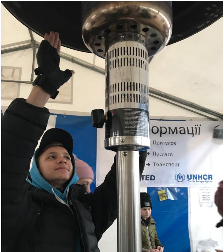
At the Palanca bus station, heater are installed in the waiting area
